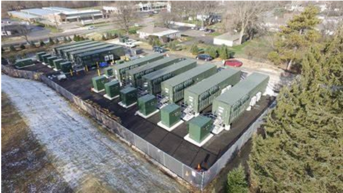
PLATE 1, TYPICAL BATTERY ENERGY STORAGE SYSTEM
